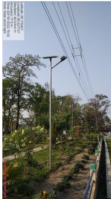
Figure 5: 30-Watt Solar Street Light Installed in the Campus
